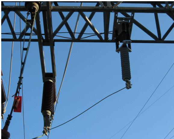
69kV HV Station Class Coupler
